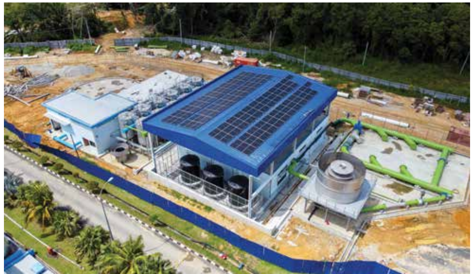
54kw solar panel installation at Sultan Iskandar Water Treatment Plant extension project.
