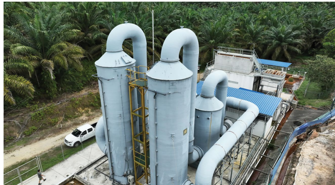
PRS System, Air Stripper and Gas Scrubber with Treatment Capacity up to 500ppm of ammoniacal nitrogen content
